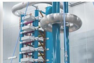
High Voltage Substation Equipment
